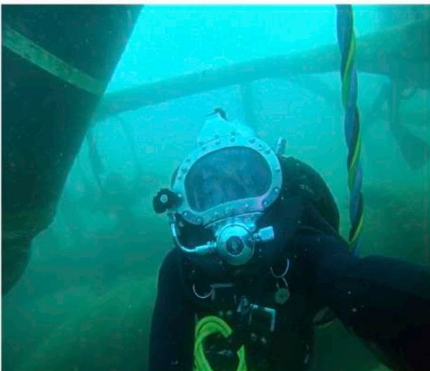
Our Certified Commercial Divers following all safety protocols performed underwater ultrasonic thickness gauging of pipes as well as underwater magnetic particles destructive tests on specific points. They also performed surveys on the hoses, couplings, and flanges of the pipeline system.
