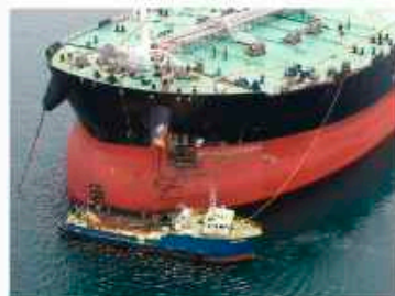
MAJOR AFLOAT STRUCTURAL REPAIRS Renewal of sections of her bulbous bow and forepeak tank.
