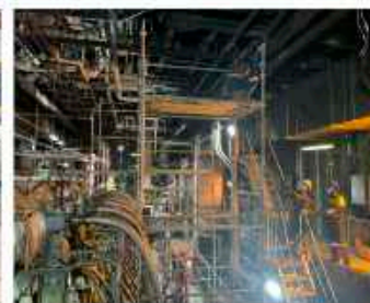
MAIN ENGINE FIRE REPAIRS Complete repair of container Vessel at Cristobal, Panama.
